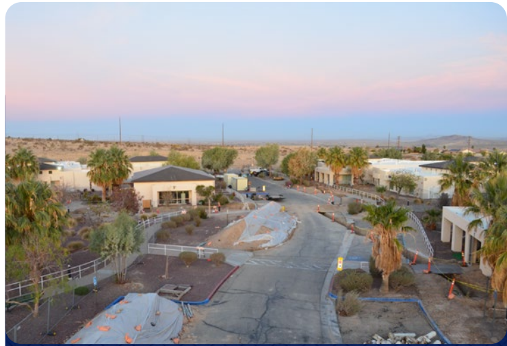
The hydronic piping repair to the DOM buildings is a large maintenance project currently being completed at the Home.
