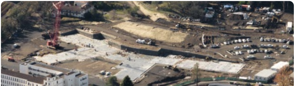
Ready for walls, a view of the foundation of the new SNF.
